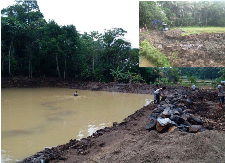
Before and during construction (funded by the 2017 Village Fund, amounting to IDR 203,000,000)
